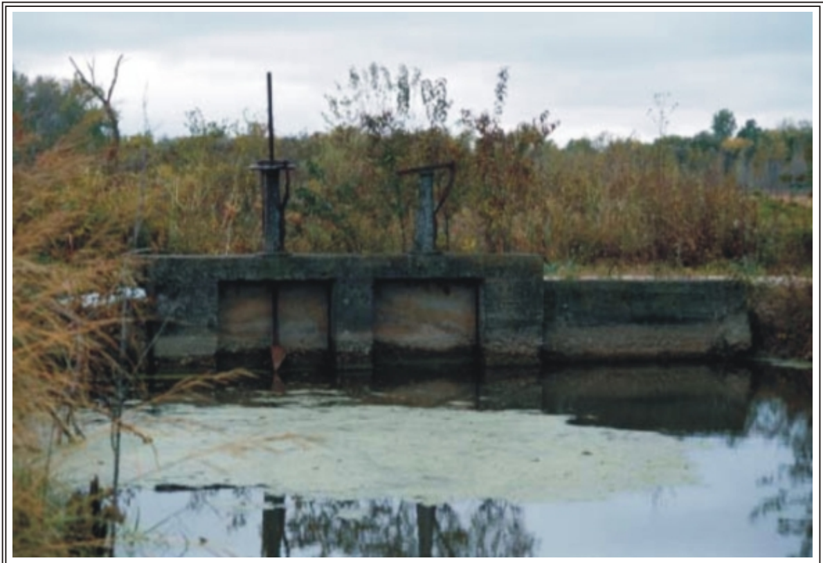
Figure 32. View South at Water Control Structure #1.
